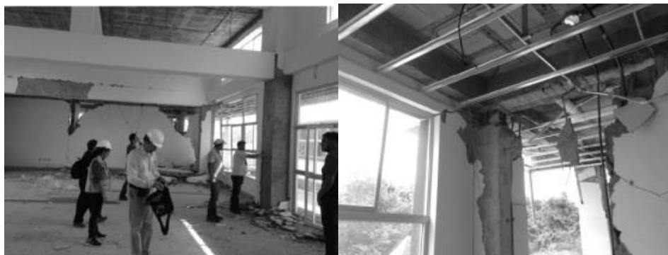
Figure 4.1. Schools damaged by the earthquake: top (two photos): in Pedernales – left (a) shows the most of the damages are the non-structural parts, and right (b) shows a joint damage of this school. Photos: IDB.
