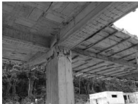
Figure 4.2 Joint damage in the school in La Siberia. This school was under construction when hit the earthquake. Photo: IDB.
