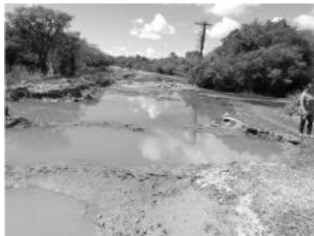
Figure 4.3. The rural path with erosions due to floods. Source: Salvatierra (2016)
