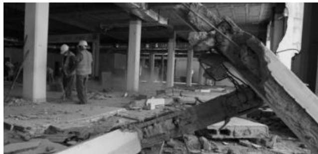
Figure 4.7. Damaged Building of Supreme Court in San Pedro Sula. Photo: HRN La Voz de Honduras
