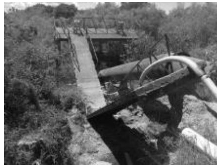
Figure 4.5. Flood control facility damaged during 2015-2016 ENSO. Source: Salvatierra (2016)
