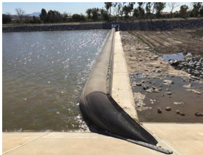
Figura 11: Dique de goma completamente inflado (Orange County Water District, 2016)
