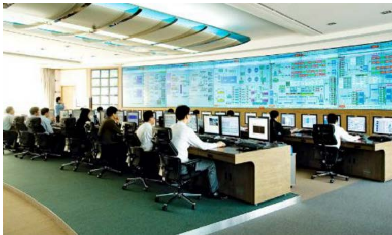
FIGURE 32: Integrated Operational Control Center for the Multi-regional Water Supply System
