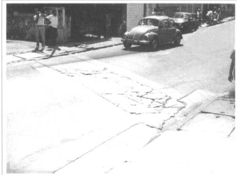
FIGURE 10.5 EXAMPLE OF CHANNEL BUILT OF CONCRETE WITH INSUFFICIENT RESISTANCE SAPOPEMBA AVENUE – SÃO PAULO
