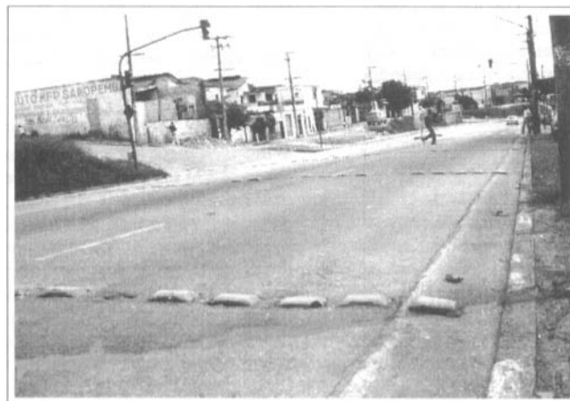
FIGURE 10.3 EXAMPLE OF LOCATION WITH STUDS DAMAGED OR WRENCHED OUT BY VEHICLES SAPOPEMBA AVENUE – SÃO PAULO
