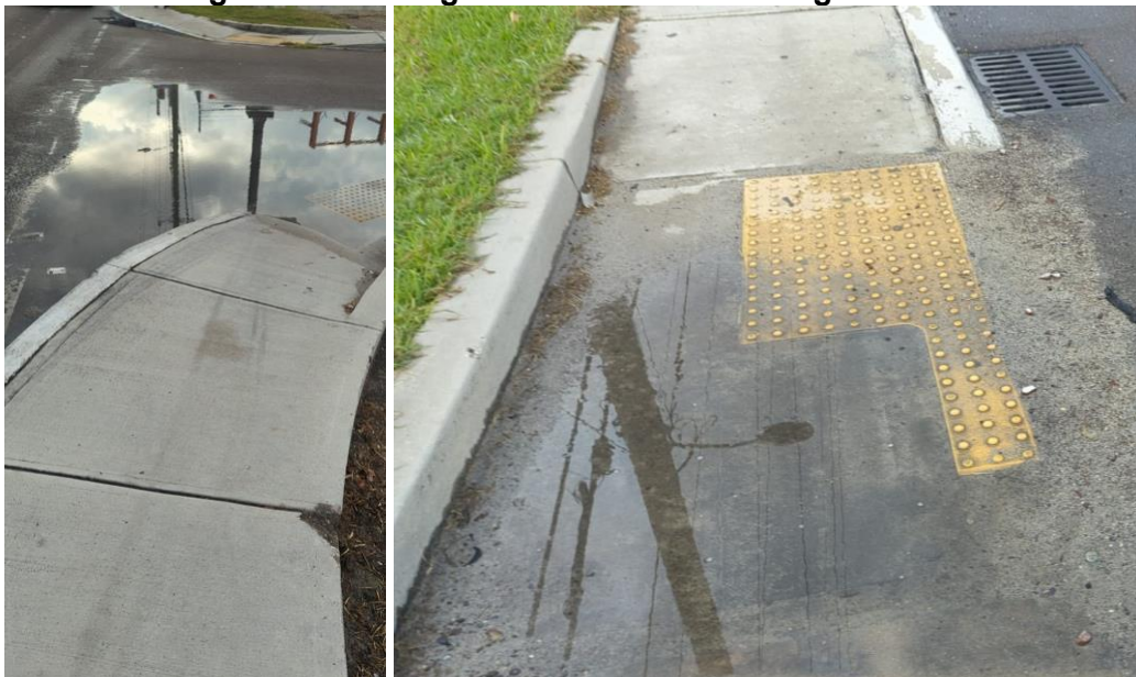
Figure 8. Flooding near Doris Johnson High School
