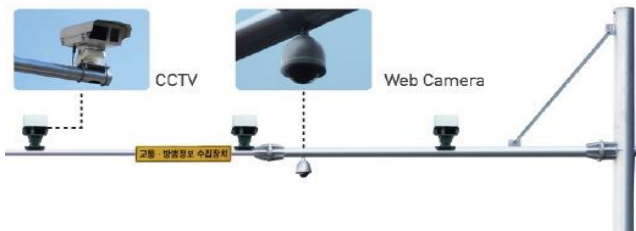
Figure 41 Automatic vehicle identification system
