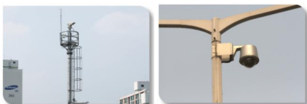
Figure 36 Closed circuit television (left) and vehicle detection systems (right)
