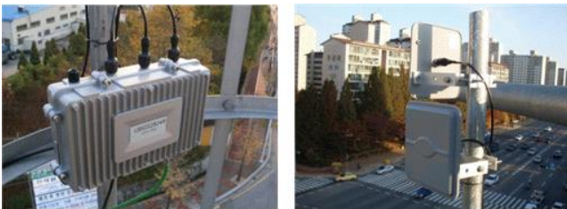
Figure 29 RSE (left) and antenna (right)
