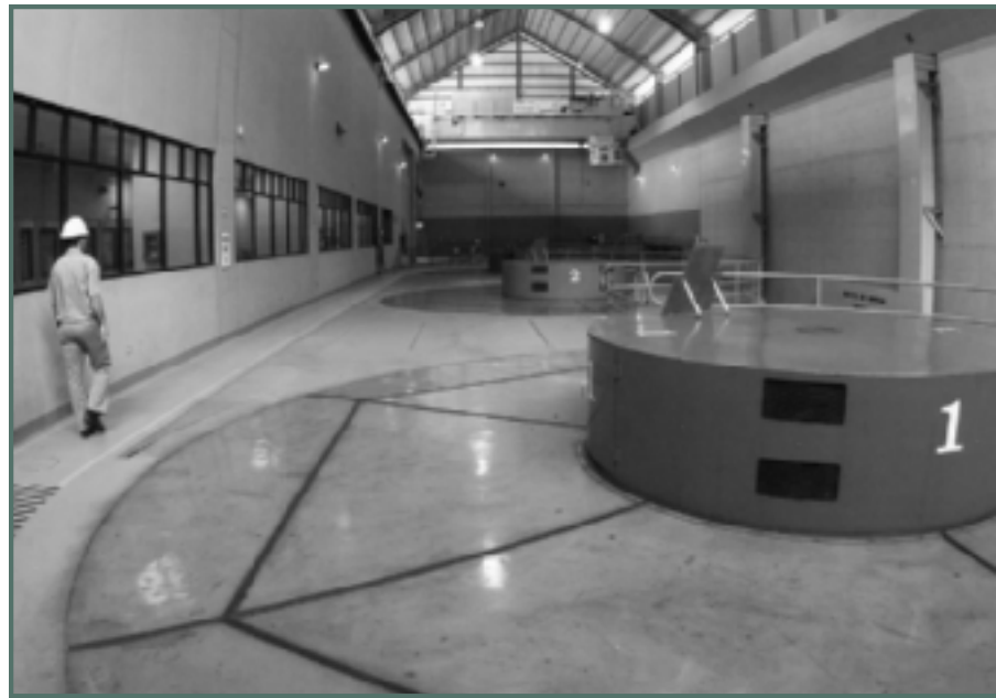
COSTA RICA • The Angostura hydroelectric power plant was built under stage III of the Electric Power Development Program to expand coverage, ensure service quality and conserve energy.
