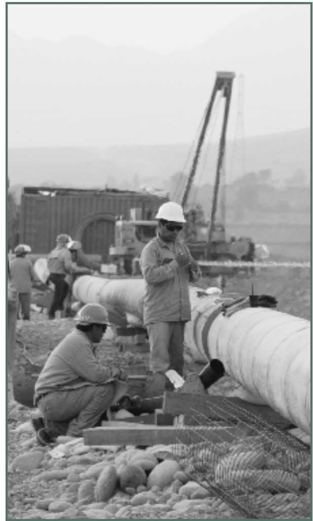
PERU • The Camisea natural gas field and pipeline distribution network is providing critical energy resources to Lima and Callao.
