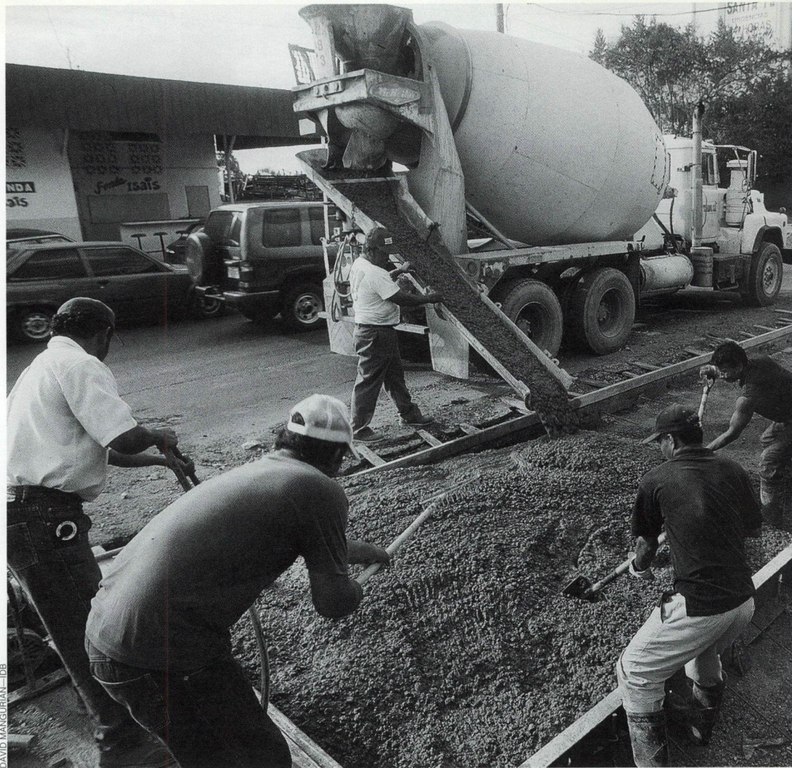
Workers in Panama City, Panama, add a fourth lane to the Avenida Simón Bolívar as part of an IDB-financed project.
