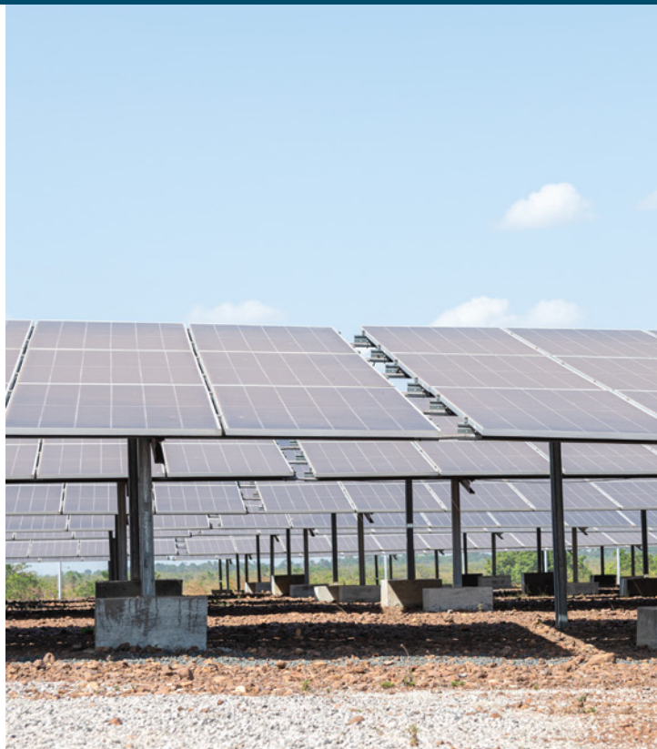
Lethem Solar PV Farm.
