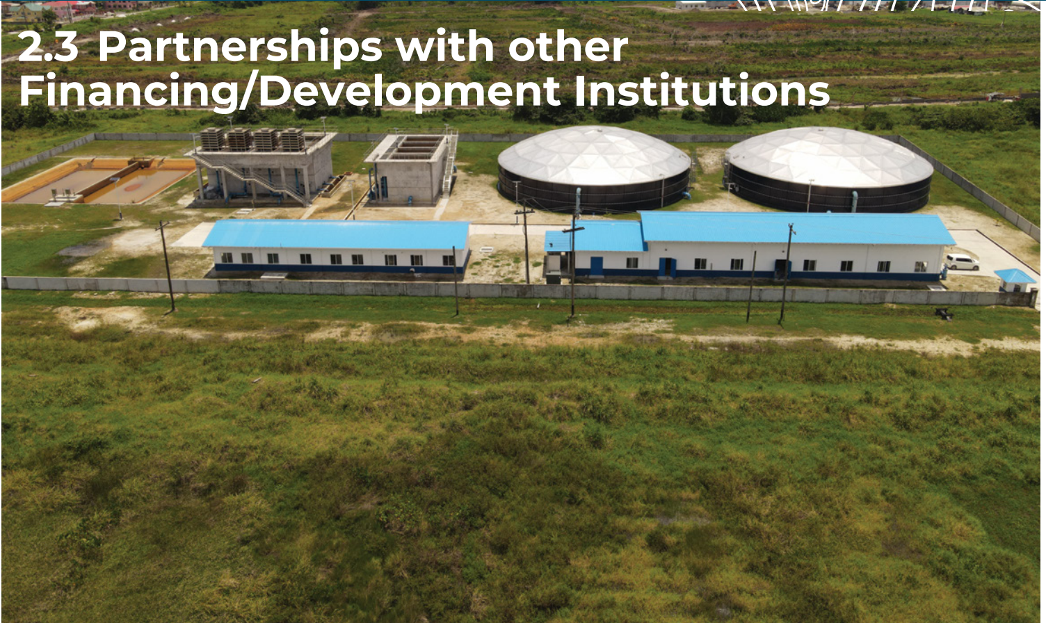
Water treatment plant constructed in partnership with the European Union at Diamond, East Bank Demerara provides improved water quality and level of service to more than 30, 000 persons.
