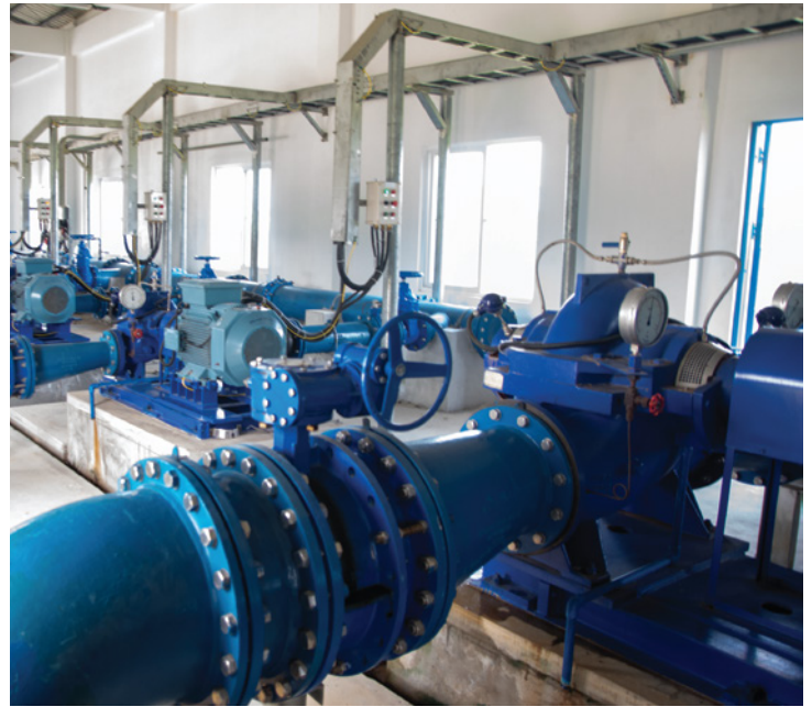
The water treatment plant at Diamond, East Bank Demerara has contributed to improved water pressure and supply.
