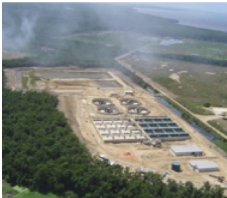
Figure 5: The Beetham wastewater treatment plant in Port of Spain is the subject of this case study on adaptation to sea level rise impacts on water and sanitation infrastructure.
