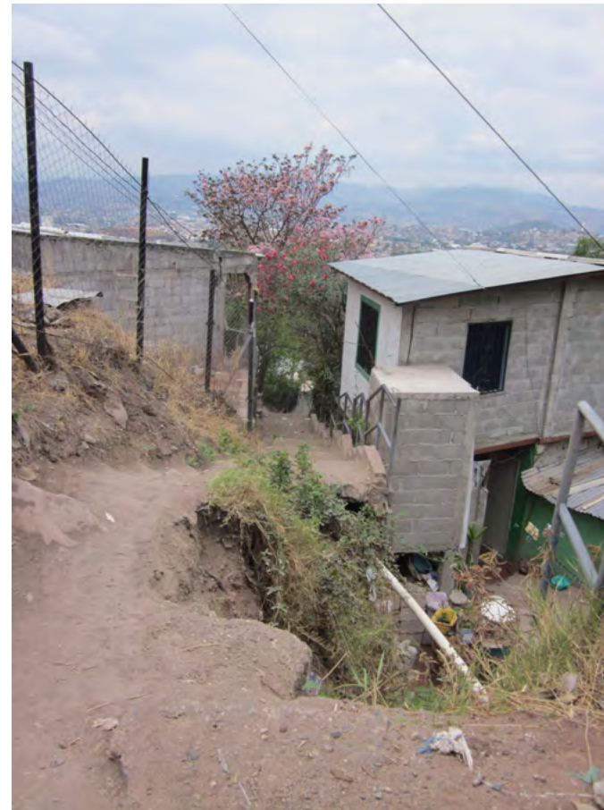
Photo 14: collapsed stairway and latrine at risk in Los Pinos
