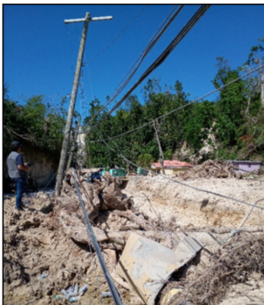
Image XIV 1: Telecommunication lines destroyed in Montego Bay
