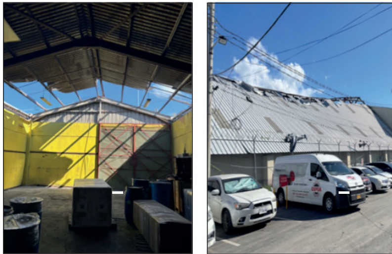
Image XI 3: Bay Roof Damage to Montego Bay Cargo Port
