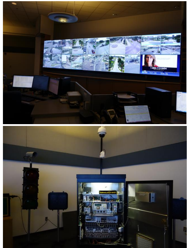
Figure 21 Traffic Management Center within OOC (source: Kwon, 2015b)
