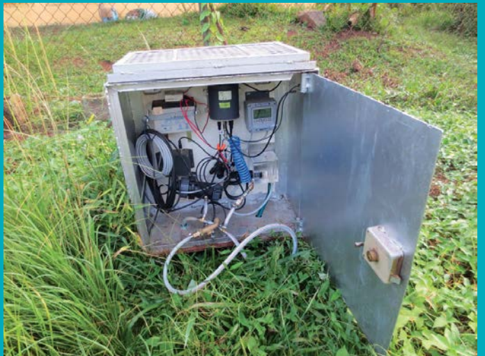
Continuous monitoring station with pressure, turbidity and free chlorine sensors.
