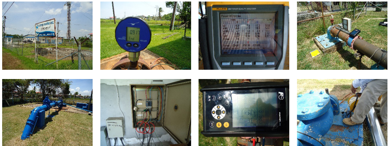
Figure 12: Field Measurements of Hydraulic and Electrical Parameters
