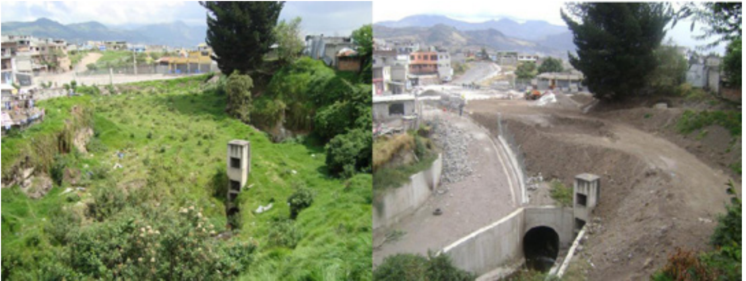
Figure 12 : Ortega Ravine project / Section 2 - Noboa Street / Left Image - Before works / Right Image - After works
