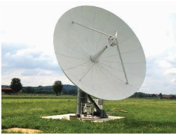
FIGURE 1.9 Example of a Satellite Antenna for a Local Hub Station
