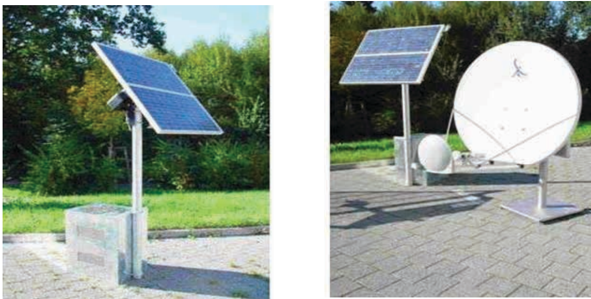
FIGURE A.8 Examples of Sun-Powered VSAT Terminals a
