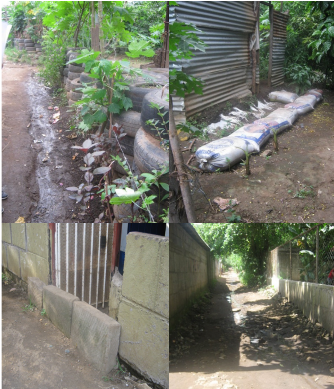
Figure C-7: Flood Prevention Barriers in the Selected Neighborhoods
