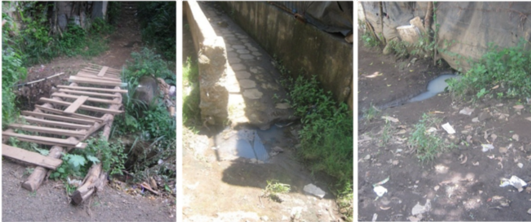
Figure C-11: Neighborhood Infrastructure in Need of Repair in the Study Communities
