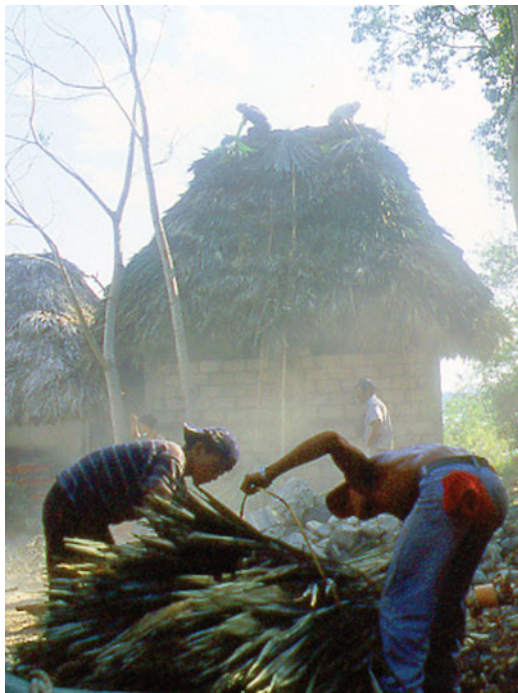
Palm thatch roofs made the traditional way turn humble restrooms into Mayan period pieces.
