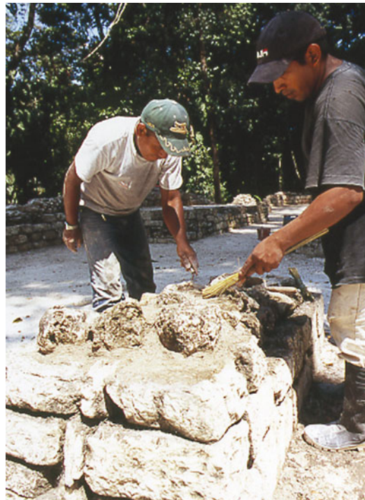
Masons occasionally experience a bad "mix," when the mortar doesn't cure properly. These workers had to dismantle previously restored walls and try again.
