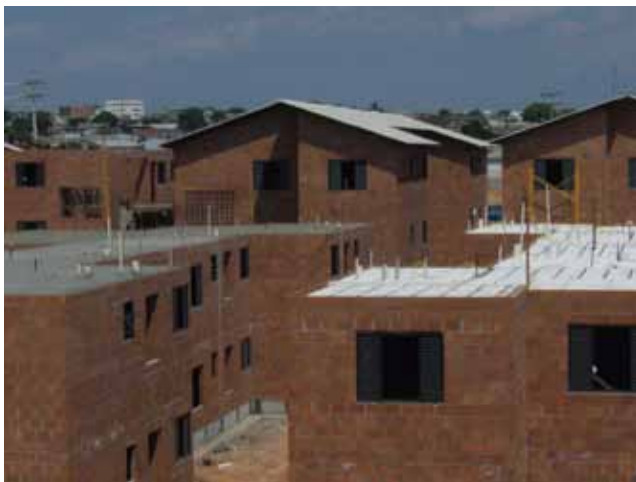
Prosamim – Construction of the new typology, with the old one in the background
